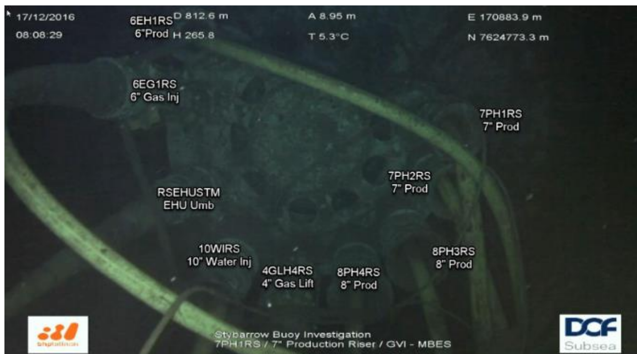
Figure 3-6: Image from ROV inspection footage showing riser entry to the base of the DTM buoy on the seabed
