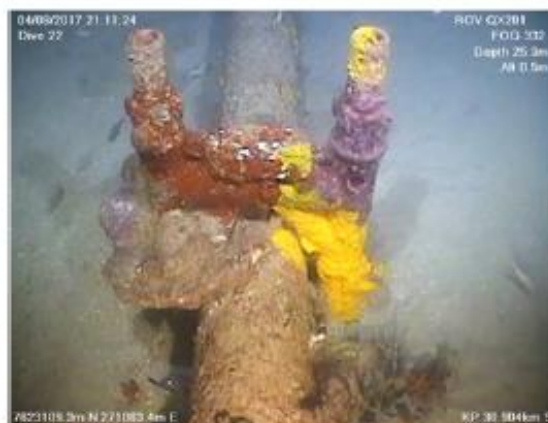
Image 2. Rock bolts secure the GEP in some sections to increase pipeline stability
