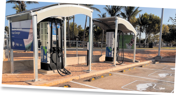
The EV fast charging station in Exmouth. Picture: The Shire of Exmouth
