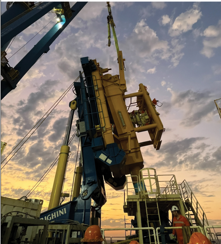
Several of the Scarborough Energy Project EPs were accepted in late 2023, including trunkline installation, with the work completed in October 2024.
