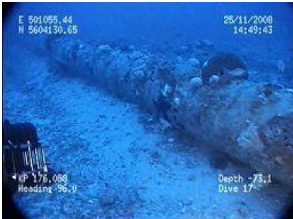
Figure 11: TGP subsea pipe and seabed
