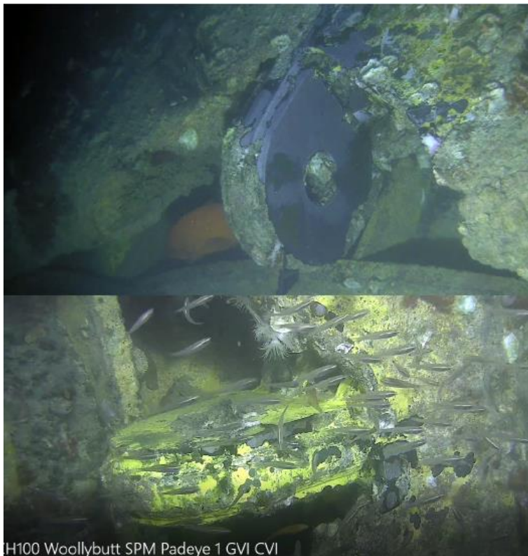
Figure 3-14: DSPM lifting lugs – Top 11 o'clock position, bottom 3 o'clock position as fallen
