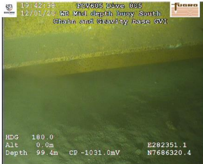
Figure 3-16: South gravity base scour on north side
