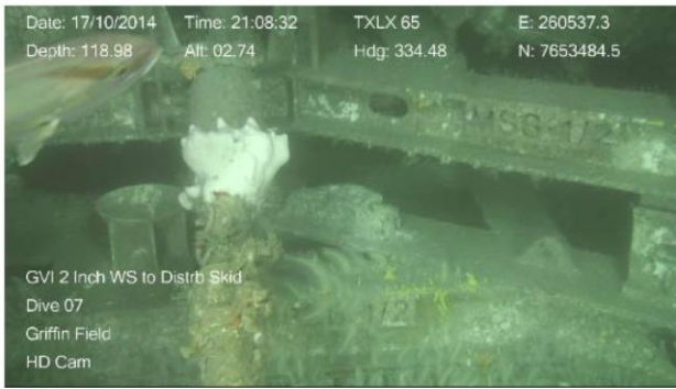
GVI 2 inch WS to Distribution Skid
