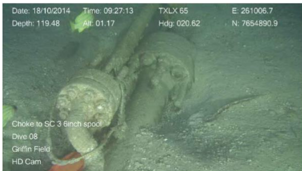
Choke to SC3 6 inch spool
