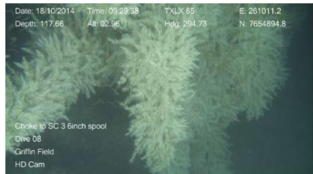
Choke to SC3 6 inch spool
