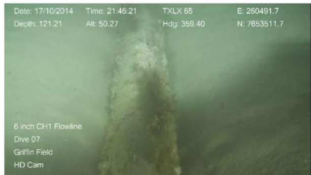
6 Inch CH1 Flowline
