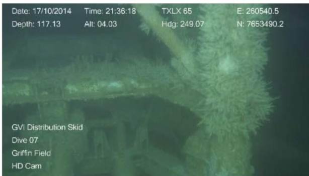
GVI Distribution Skid
