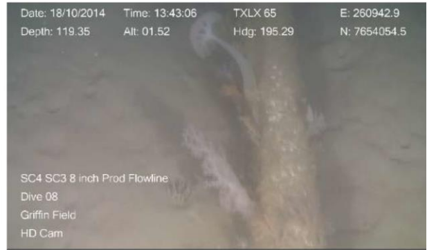
SC4 SC3 8 inch Production Flowline
