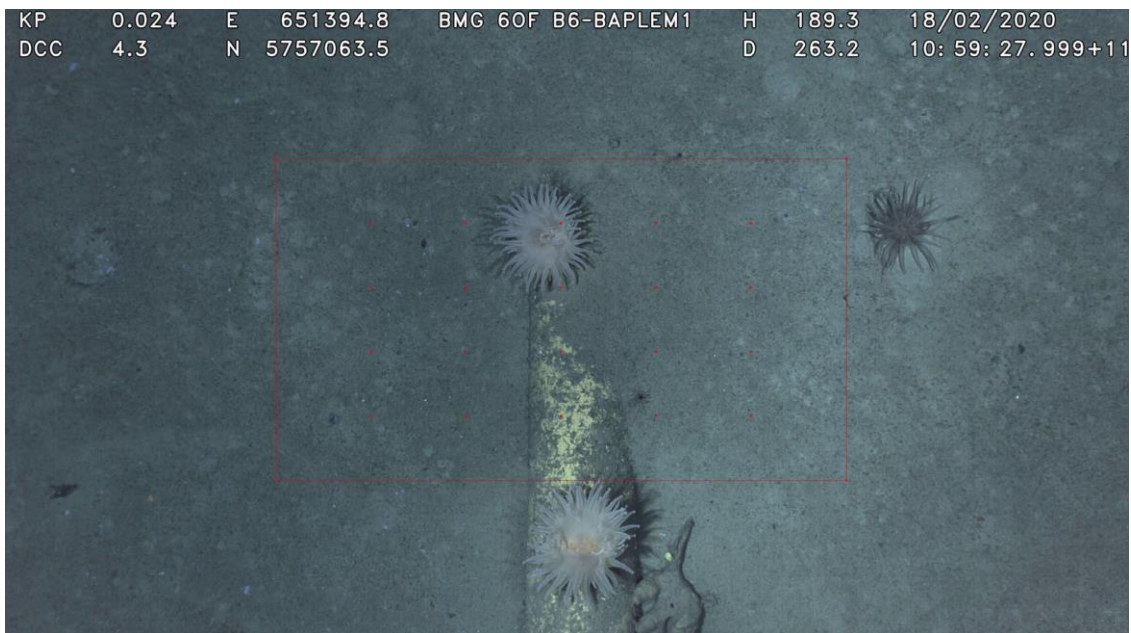
Figure 6-2 Image from 2020 GVI showing the B6 Oil flowline transitioning from above to below the seabed (Ierodiaconou et al (2021))
