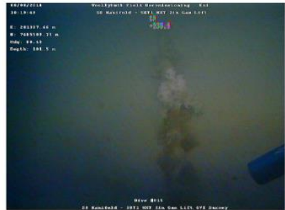
Image 2.6-02 - 2" Gas Lift - Marine Growth
