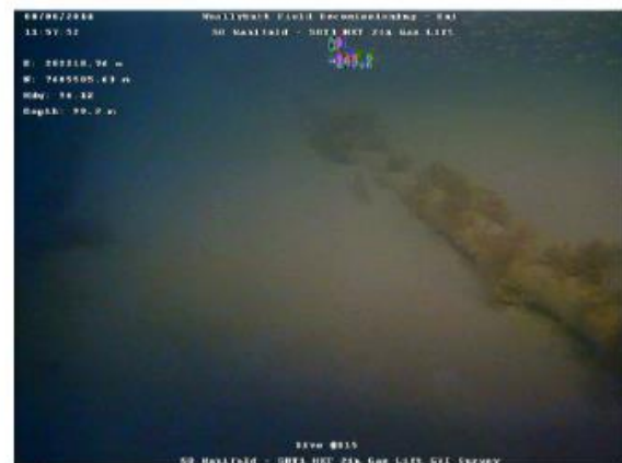
Image 2.6-04 - 2" Gas Lift - Free Span
