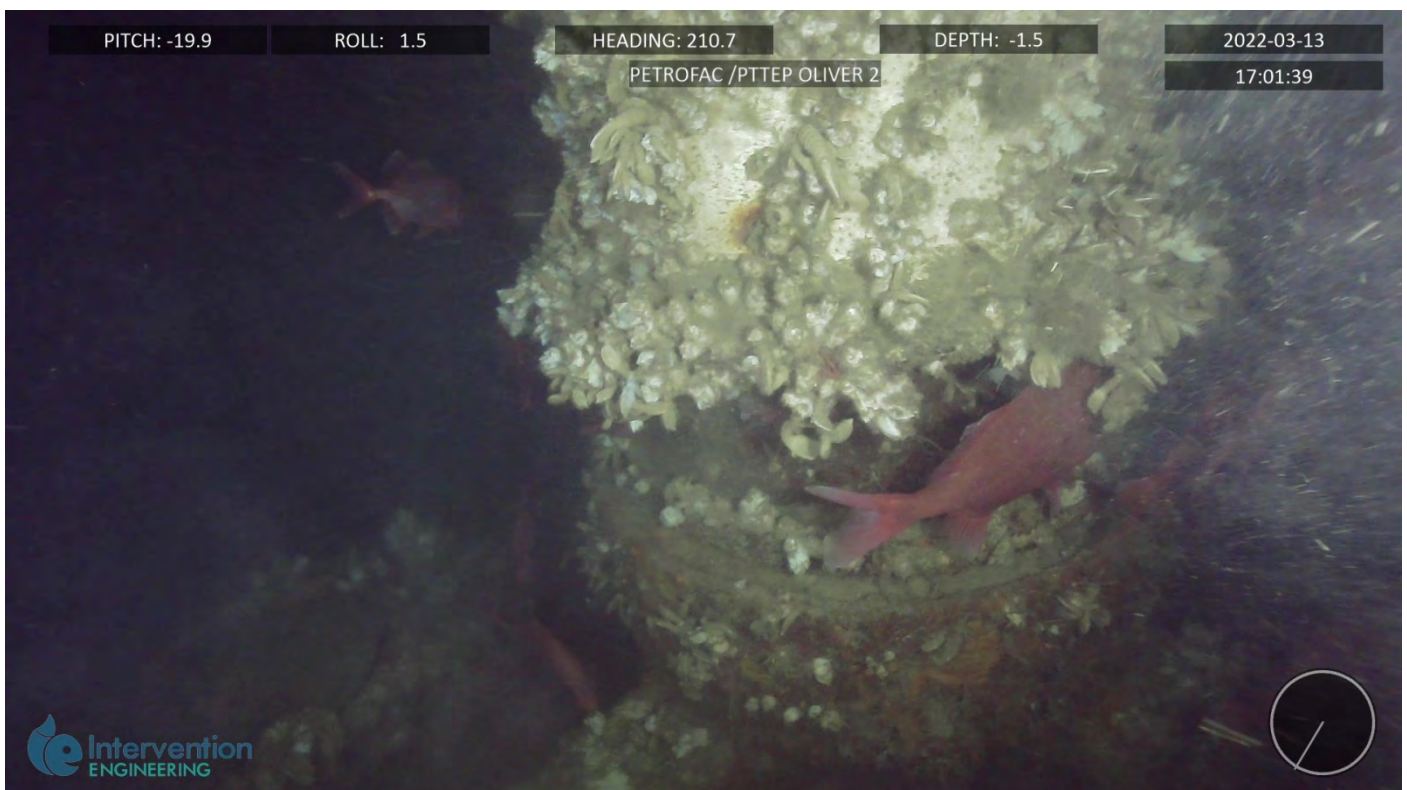
Figure 12 Oliver 2 Example of corrosion on wellhead
