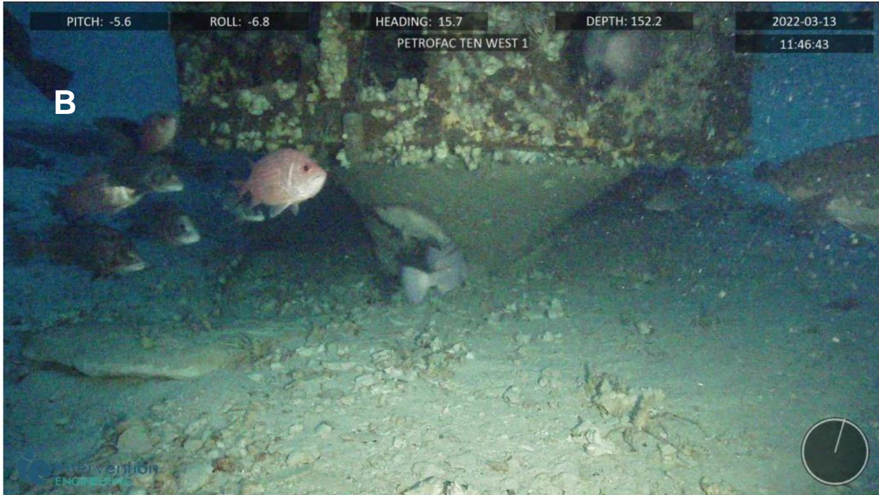
Figure 5-3: Tenacious West-1 ST1 wellhead: A - view of the top of the wellhead including guide posts and corrosion cap; B - view of scour under the temporary guide base and sign of cement returns
