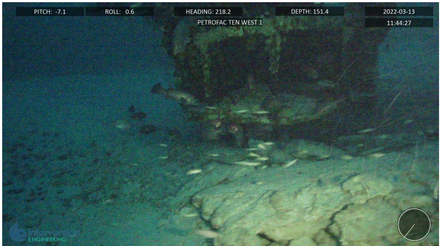
Figure 8 Ten West 1 example broken grout on seabed
