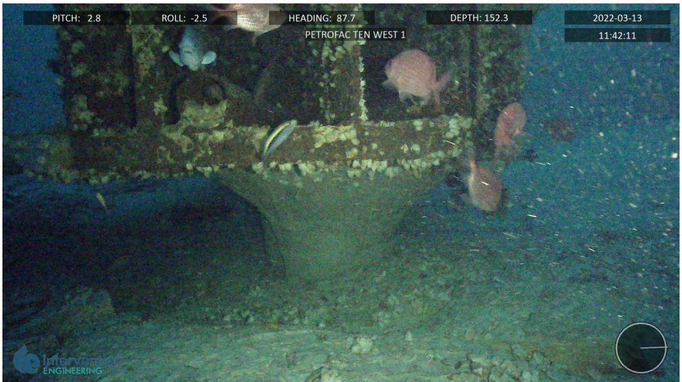
Figure 6 Ten West 1 example scour under guide base.
