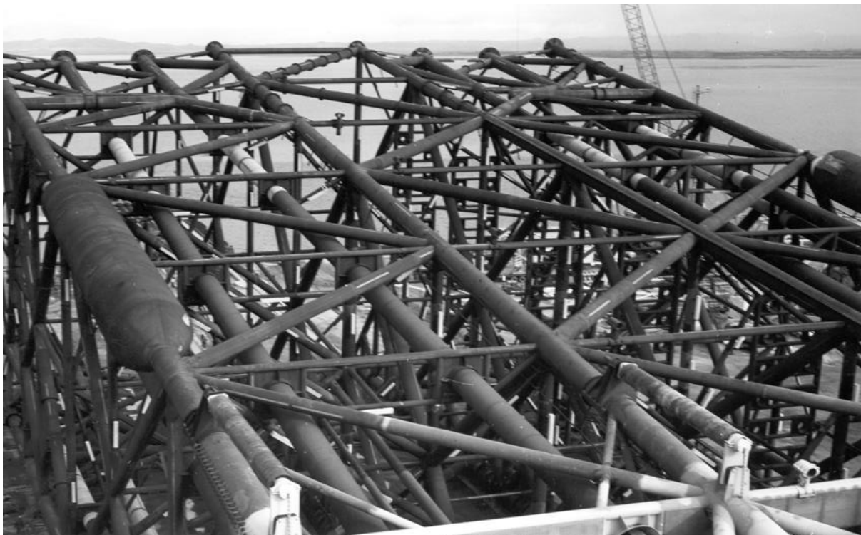
Figure 1-3 The Mackerel Steel Piled Jacket prior to installation, showing the complexity of the structure
