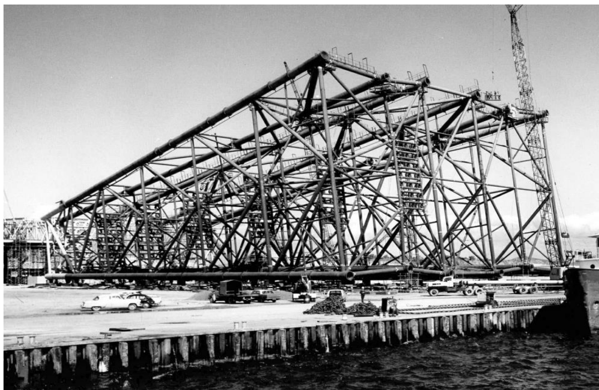
Figure 3-12 One of the Kingfish Steel Piled Jackets under construction at Barry Beach (1969)
