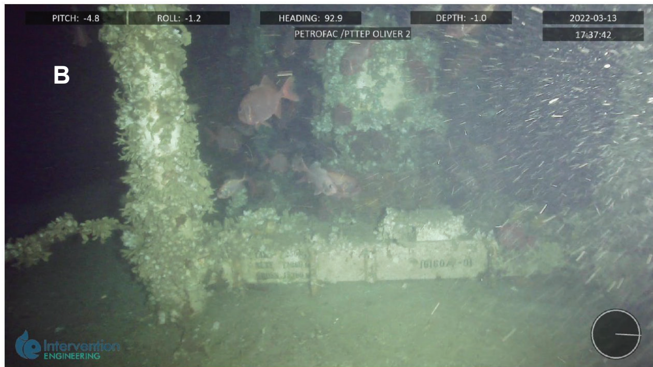
Figure 5-2: Oliver-2 wellhead: A – view of the top of the wellhead including guide posts and corrosion cap; B – permanent guide base at seabed level
