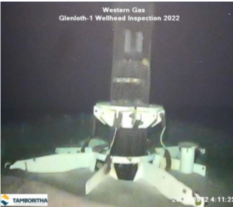
Figure 2-6: Photograph of the Glenloth-1 guide base
